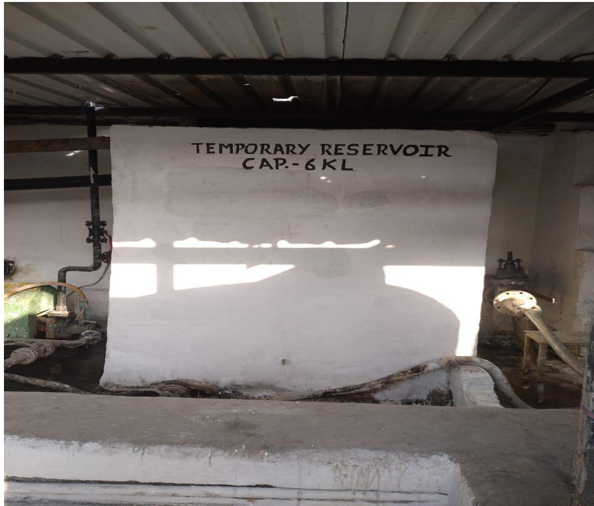
Photo-10: Reservoir for Storm Water Collection
