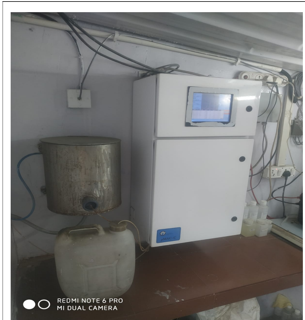
Photo-6: Online Continuous Effluent Monitoring System (OCEMS)
